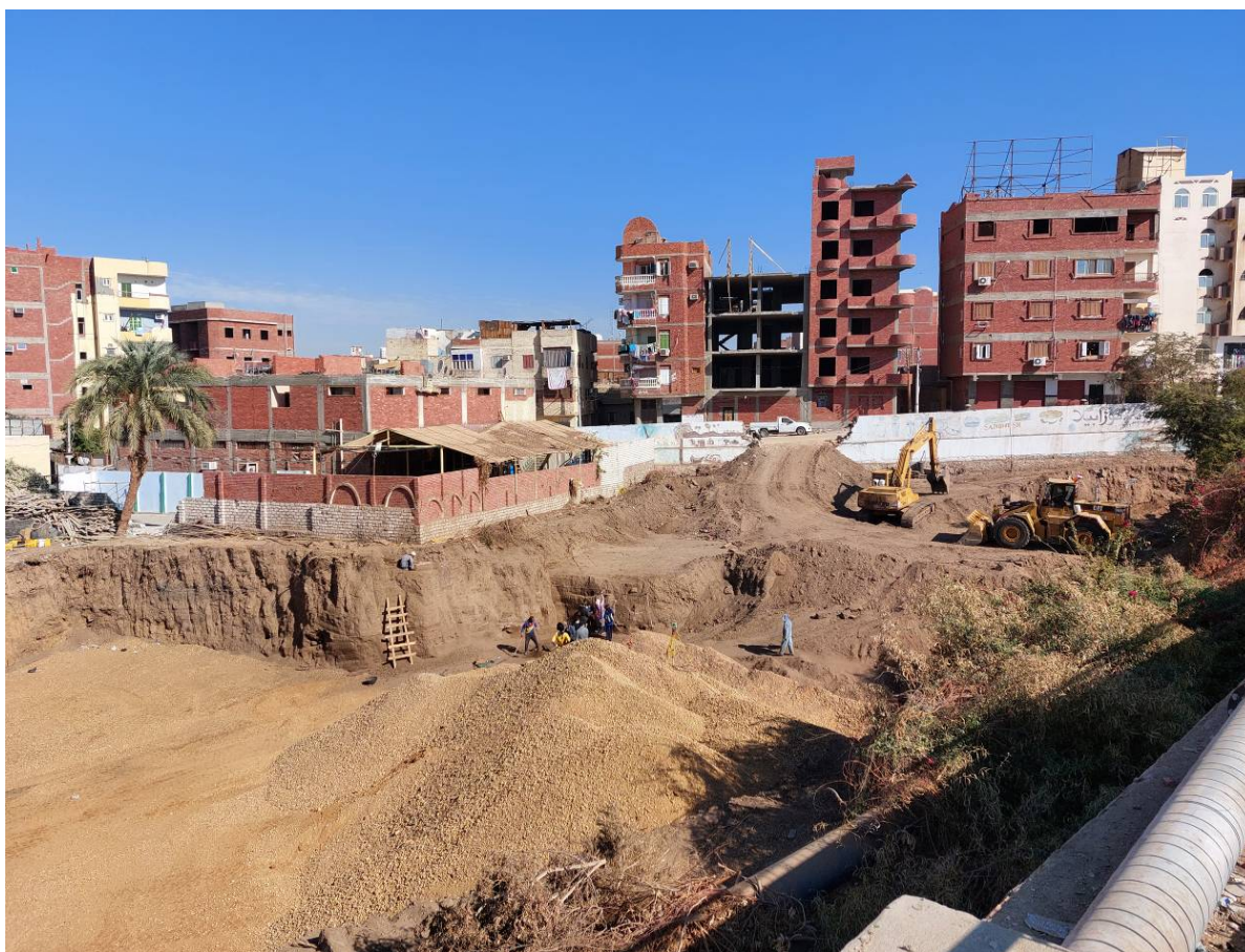
Fig. 13: Overview of Area 95 from the south-east with Sectors A and B. In the background, house under construction in former Area 93.
