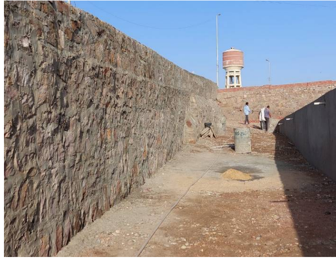
Fig. 4: Area 2: Detail of the space between the new magazine and the street to the south after backfill and consolidation and raising of the southern perimeter wall.
